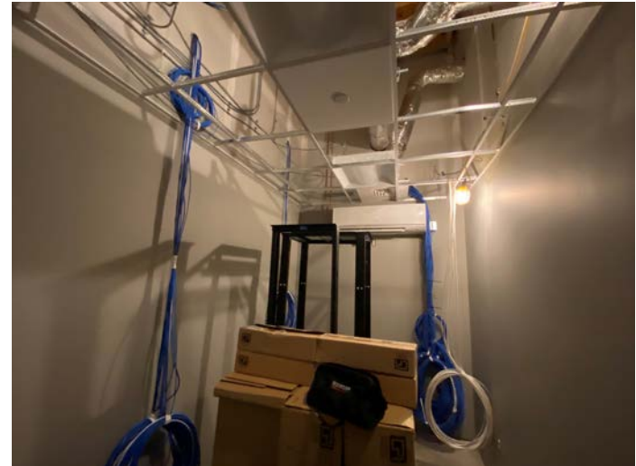
Telecommunication wire rough-in in security IT room
