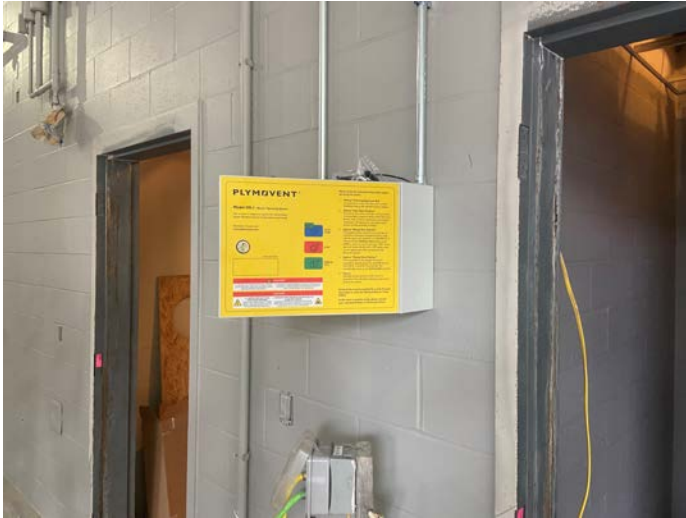
Vehicle exhaust vacuum control installation
