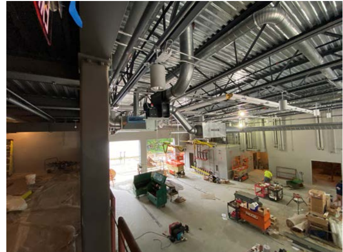
Overview of apparatus bay
