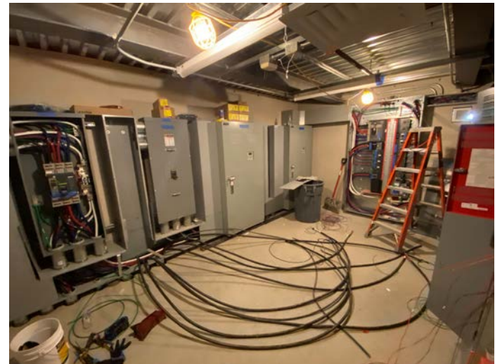
Overview of electrical room
