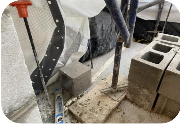
Slab edge insulation installed on east side of building (adjacent to southeastern apparatus bay)
